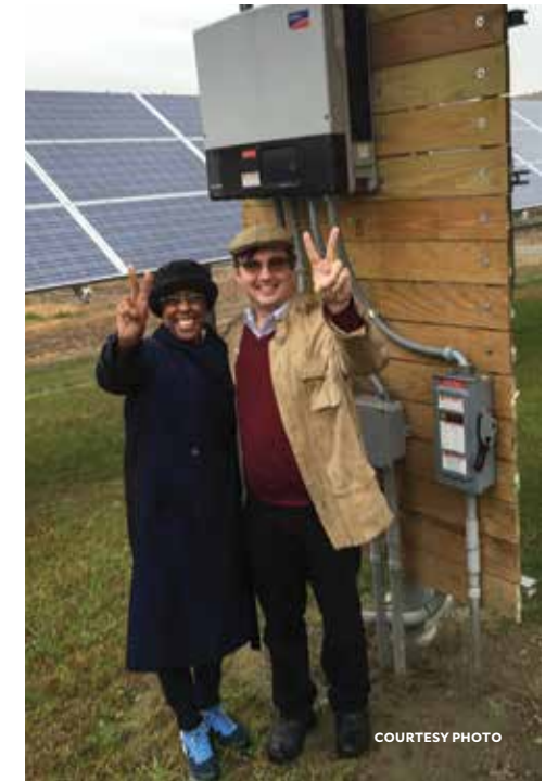
▲ Lilia Abron and her colleague John Corliss, senior vice president of PEER Consultants PC, standing in front of a solar array designed and installed by PEER at a wastewater treatment plant in Connecticut.
