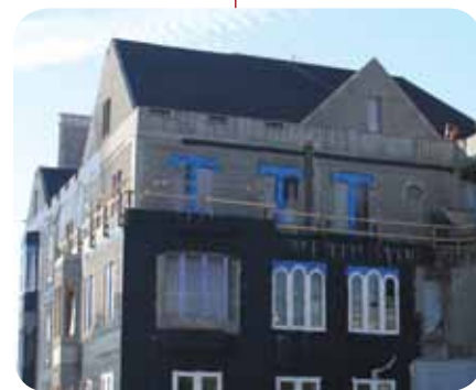
APRIL 2010 Construction began on Preston M. Green Hall, the third building in the new state-of-the-art engineering complex (see p. 32)
